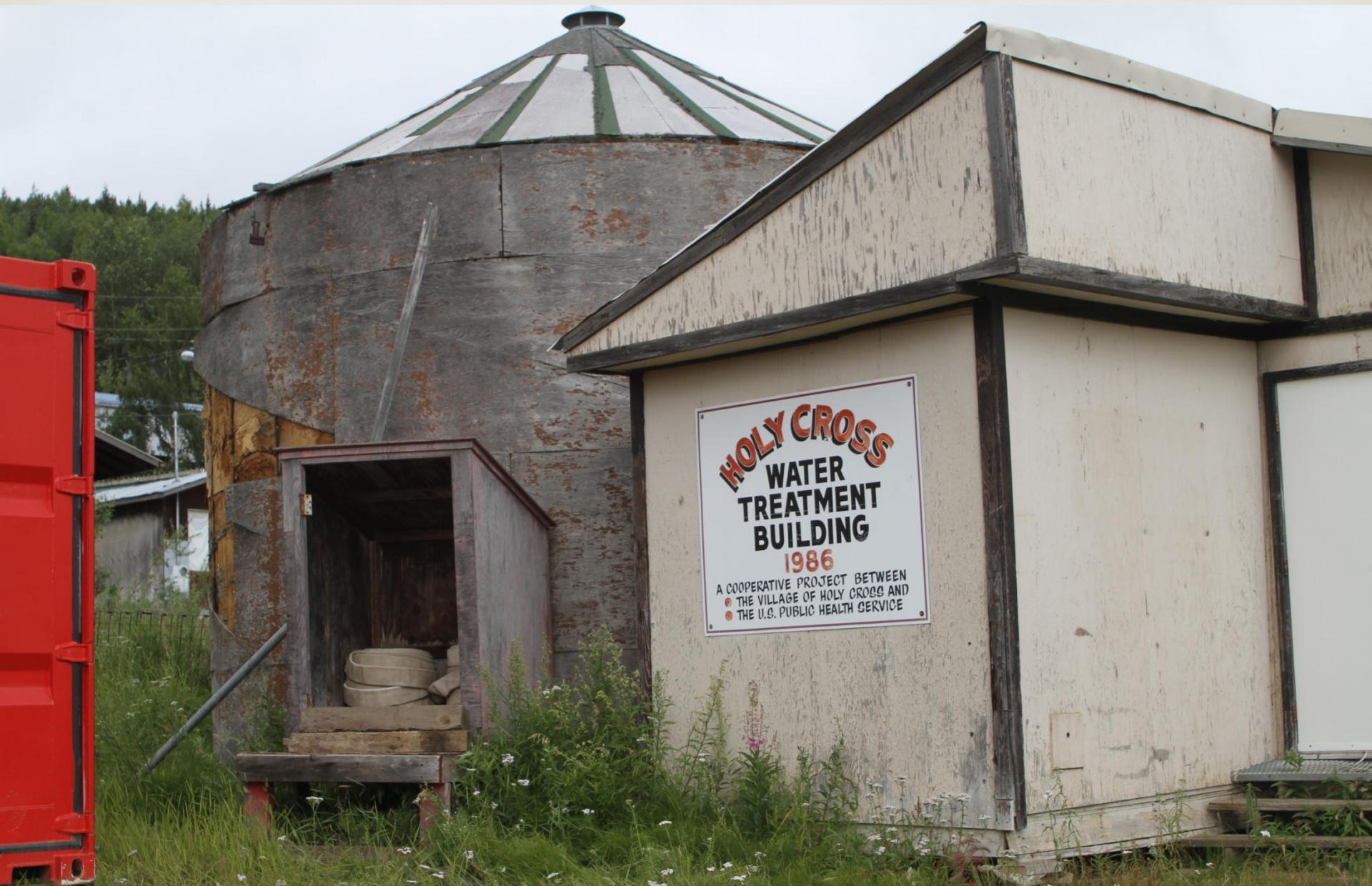
Water tank must be maintained at 42° year around. (winter -50°) Biomass residual heat is ideal
