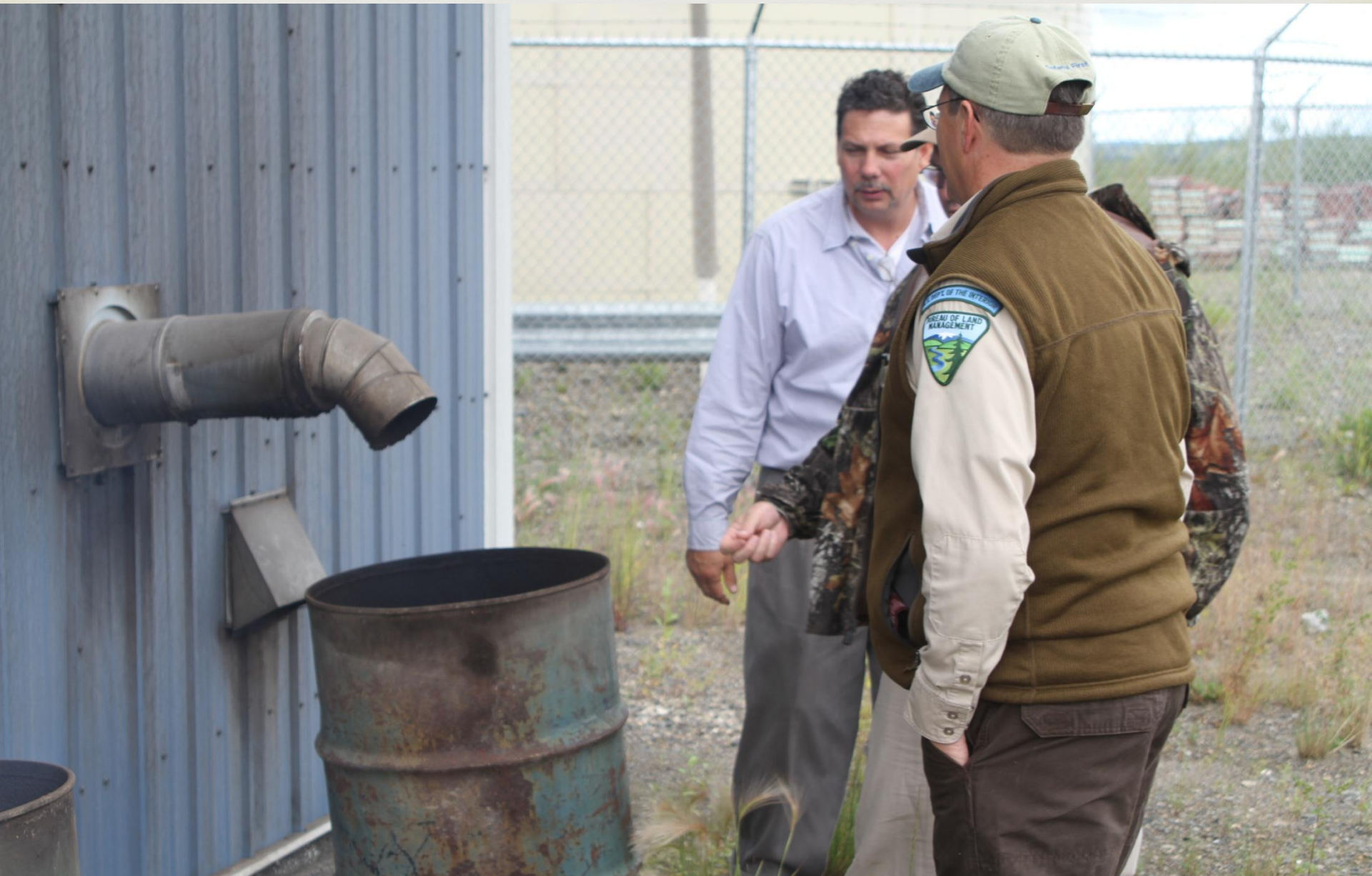
Exhaust from Garn Boiler is clean and cool. City Manager, BLM Field Manager. Bear is a key player with other communities to promote biomass use and the benefits of networking to other Native Villages.
