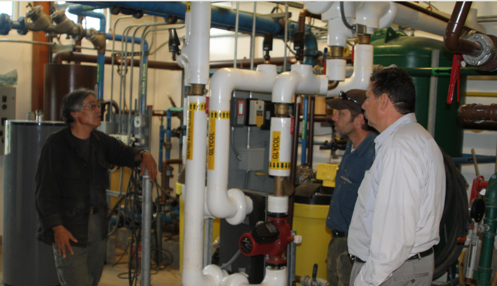
Local Operator, BLM Forester, City Manager. Heat exchange in washateria. Most villagers bring laundry to washateria/ community building. Showers are also available here. City Manager Bear Ketzler is a leader in the larger native community in promoting the use of biomass through his own network connection. Tanana will install one more boiler this year to heat the city offices and the teacher housing and 3 more next year to heat the school. Biomass power for the school will be next.
